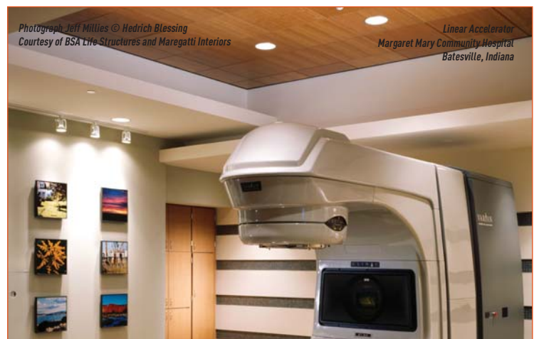
At Margaret Mary Community Hospital in Batesville, Indiana, an American cherry ceiling serves as a "positive distraction" for patients undergoing a procedure in the Linear Accelerator Suite.
